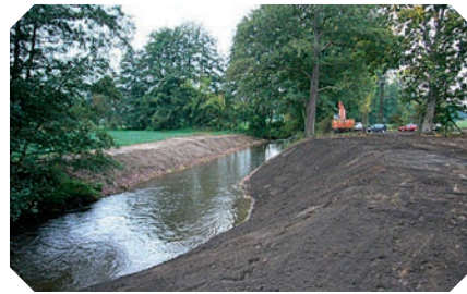
Nuthe-Wehr Pumpstation Zerbst (nachher)
